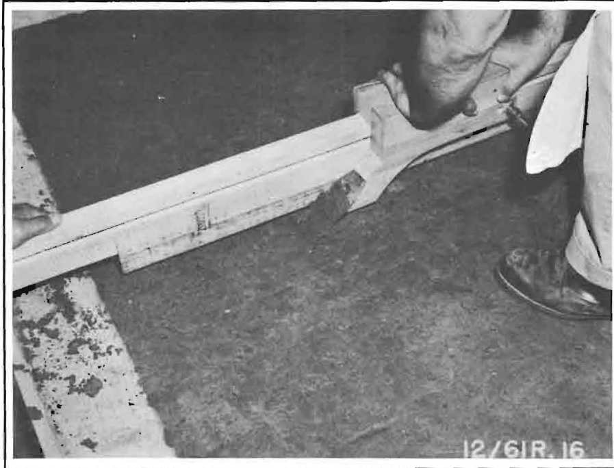
Figure 9. Subgrade planer devised for leveling the subgrade surface to provide uniform support for the test slabs.
