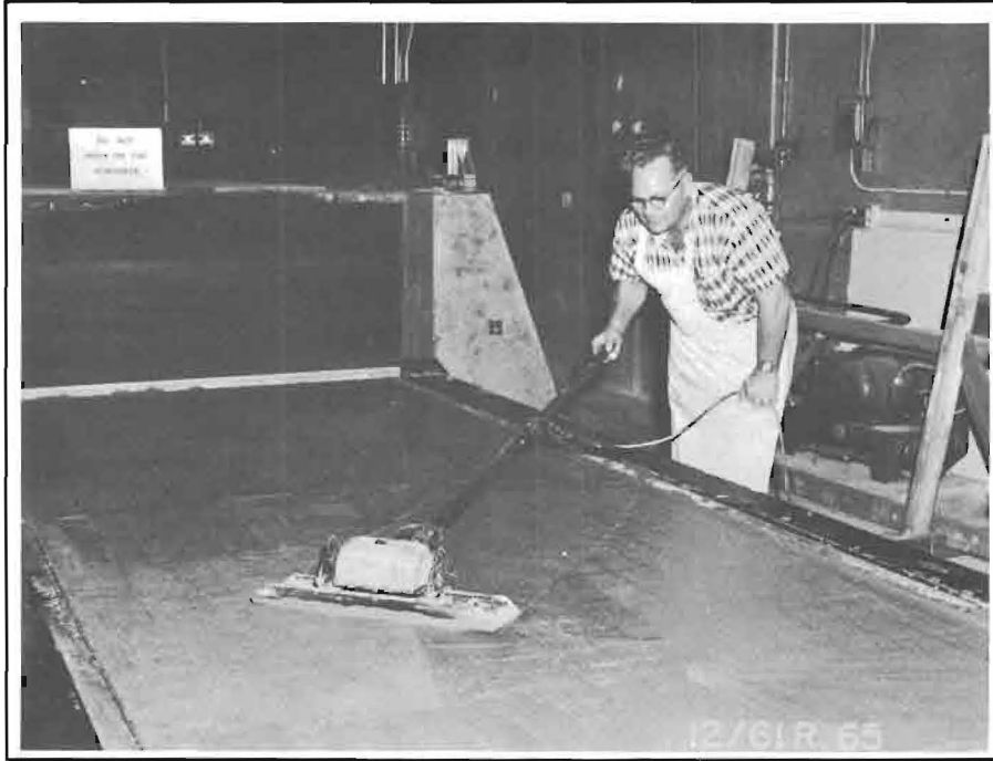
Figure 17. Plate-type vibrator being used to consolidate the concrete during construction of the test slabs.
