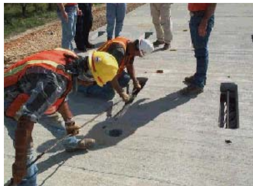
Figure 4.29 Strands will be threaded through the stressing pockets from the central panels
