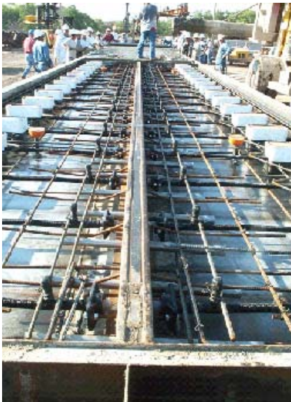
Figure 4.12. Small boxes/inserts are placed in for preparing access pockets of joint panel mold
