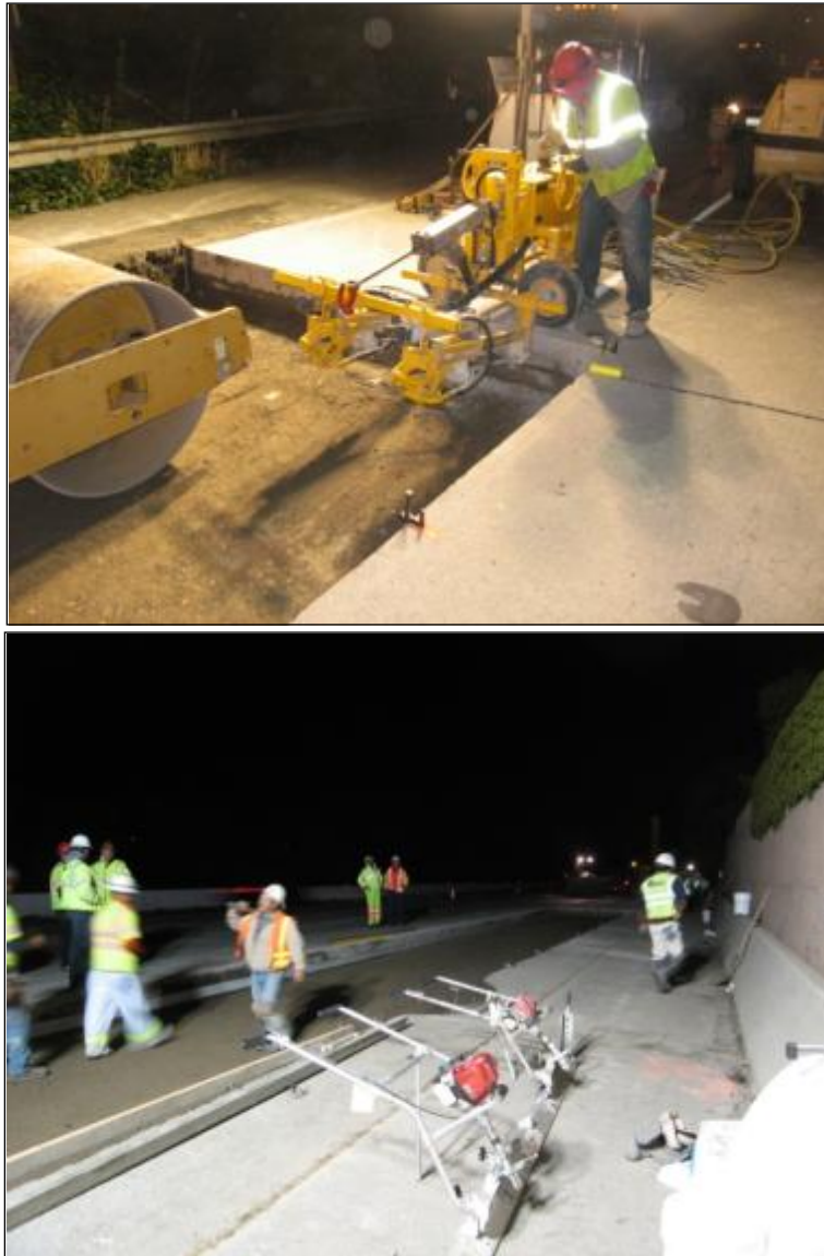
Figures 11-12 – Drilling dowel slots, placing joint filler material and setting grade for LCB-RS
